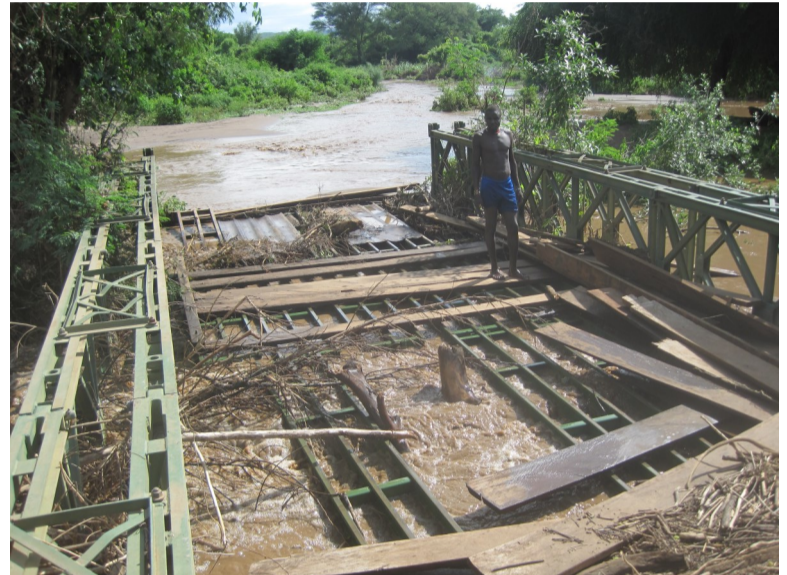
Bridge during floods showing missing grates.
